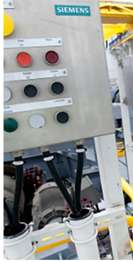
Figure 11-14 Conductors routed in raceways
