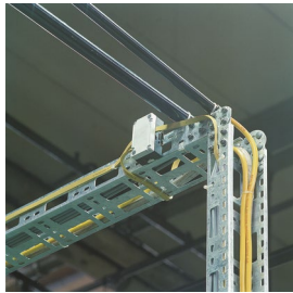
Figure 11-19 Example of exposed cables
