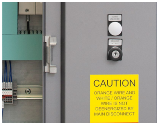
Figure 13-18 Example of safety sign for disconnecting means
