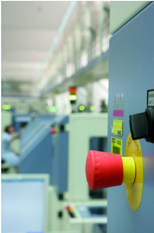
Figure 10-13 Example of an EMERGENCY OFF pushbutton in the application
