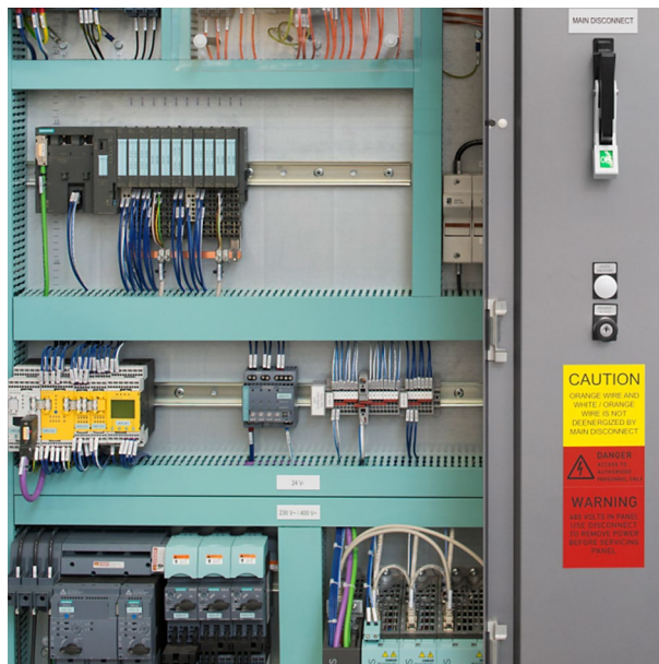
Figure 13-9 Example of warning information on the industrial control panel enclosure
