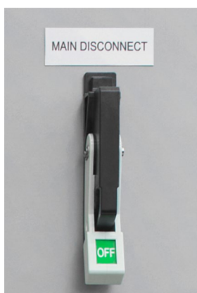
Figure 13-21 Toggle lever for main disconnecting means
